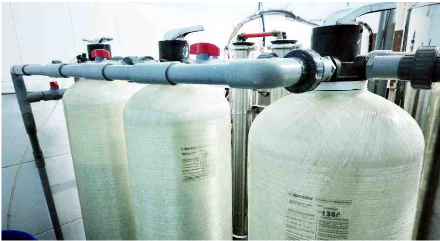
Brine residue goes into tanks for disposal.
