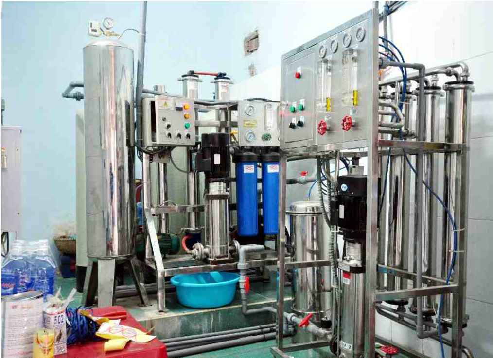
Water purifying plant at Ha Loi.
