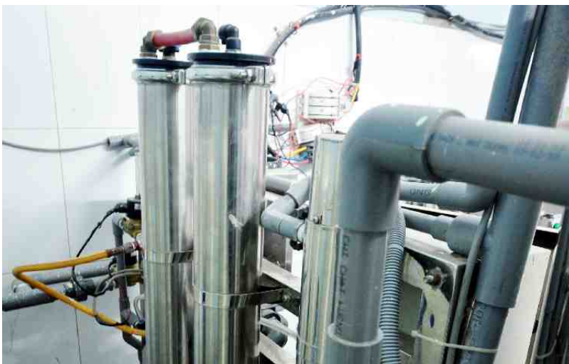
Cylinders with water softener.
