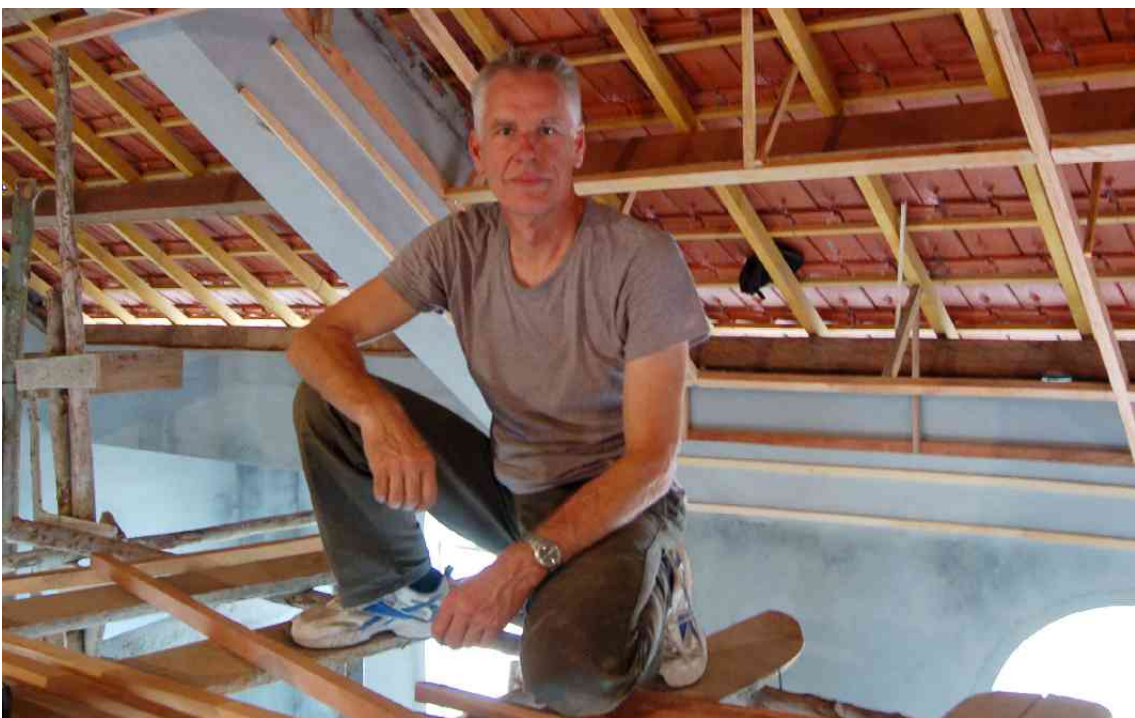
Gaps in the working platform are "normal".
