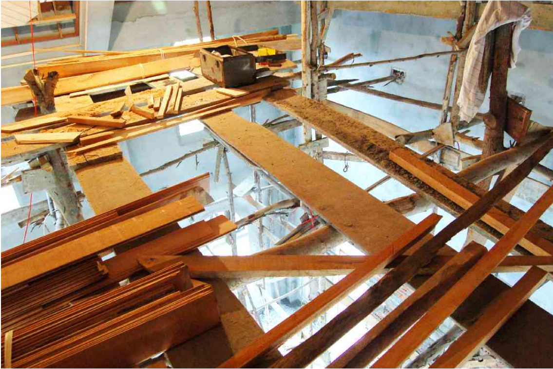
Gaps in the working platform are “normal”.
