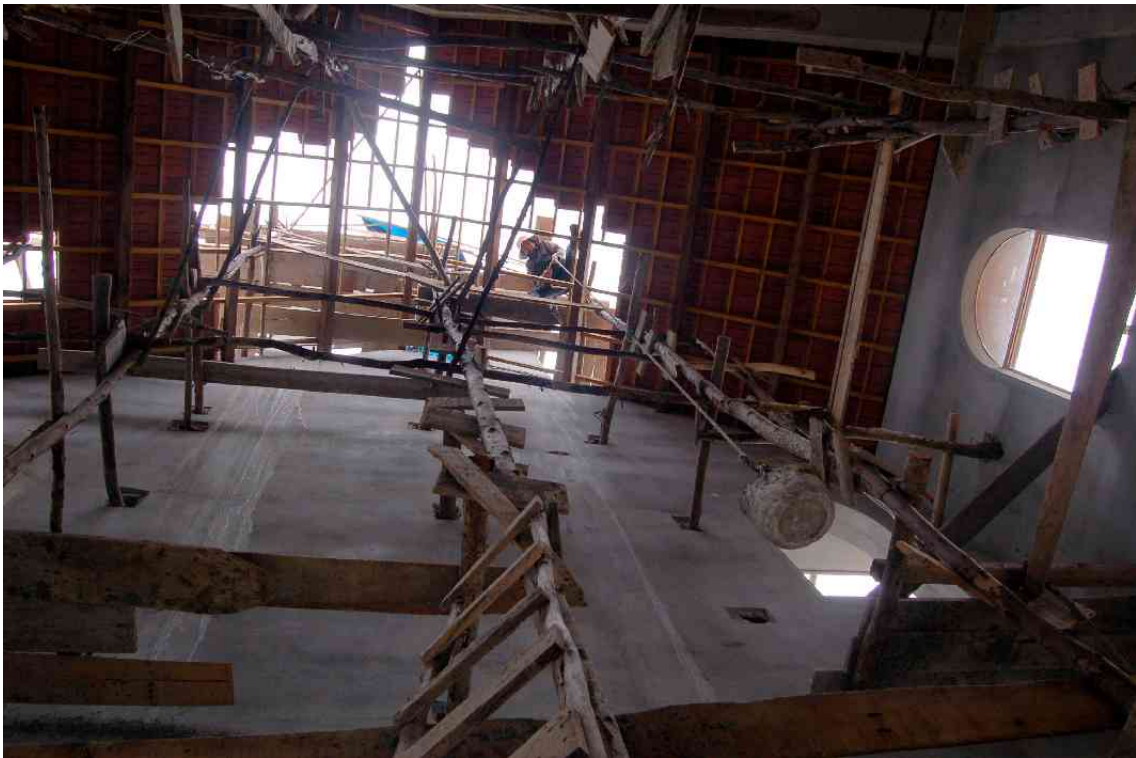
A worker at the top of the pole ladder pulls up a bucket of mixed mortar by rope.
